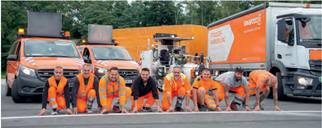
SWARCO Road Marking Systems' striping experts at work on the Digitrans test track in St. Valentin
